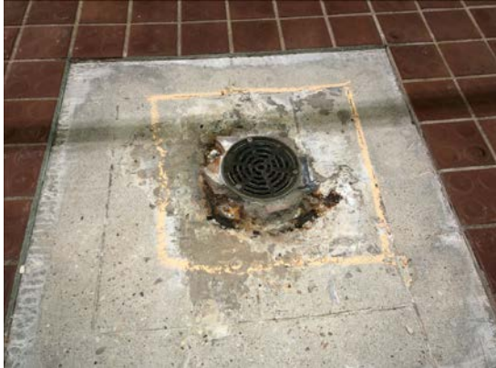
Photo 2: Delamination at Tile Removal Area C
