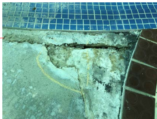
Photo 10: Concrete delamination at expansion joint
