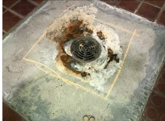
Photo 3: Delamination at Tile Removal Area D
