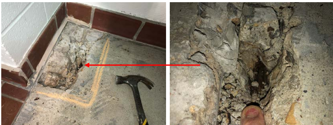
Photo 1: Delamination at expansion joint below Tile Removal Area B
