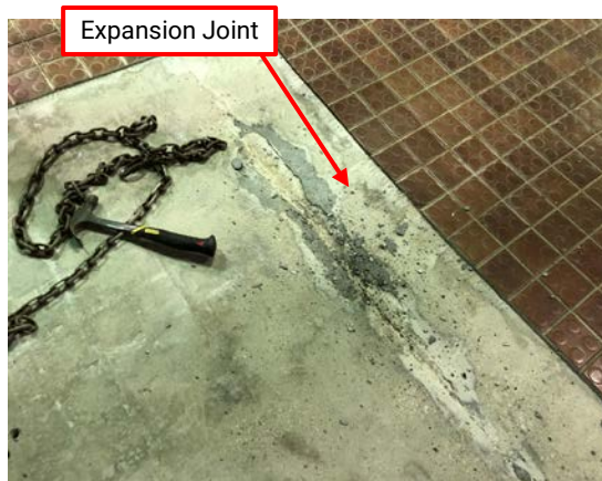
Photo 4: Unbonded grout at expansion joint
