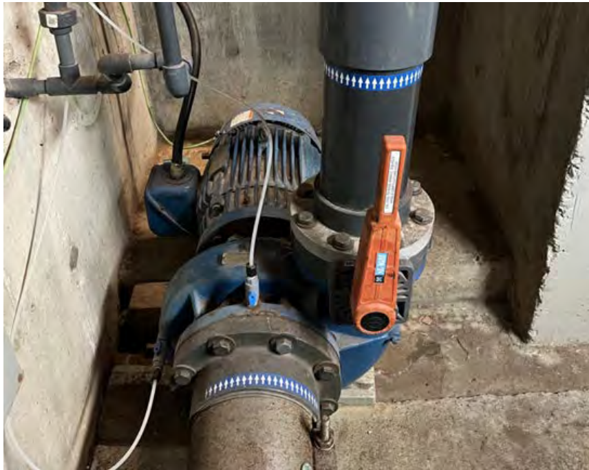
Harbour Pool Main Pump
