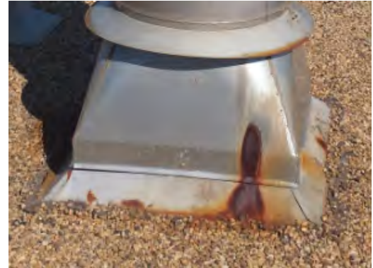
Figure 2: Surface Corrosion at B Vent Base Flange
