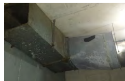
Figure 7: Exhaust Fan Hole @ Duct
