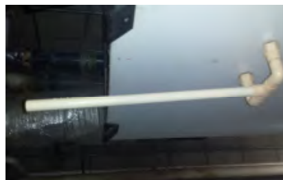
Figure 6: HRV condensate pipe
