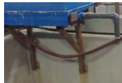
Figure 5: Corrosion @ Hopper Support
