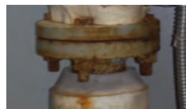
Figure 6: Glycol Leak @ Flanges
