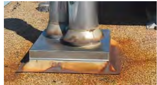
Figure 3: Surface Corrosion at Boiler Flue Base Flange
