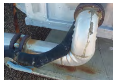
Figure 7: Alum. Jacket Deterioration
