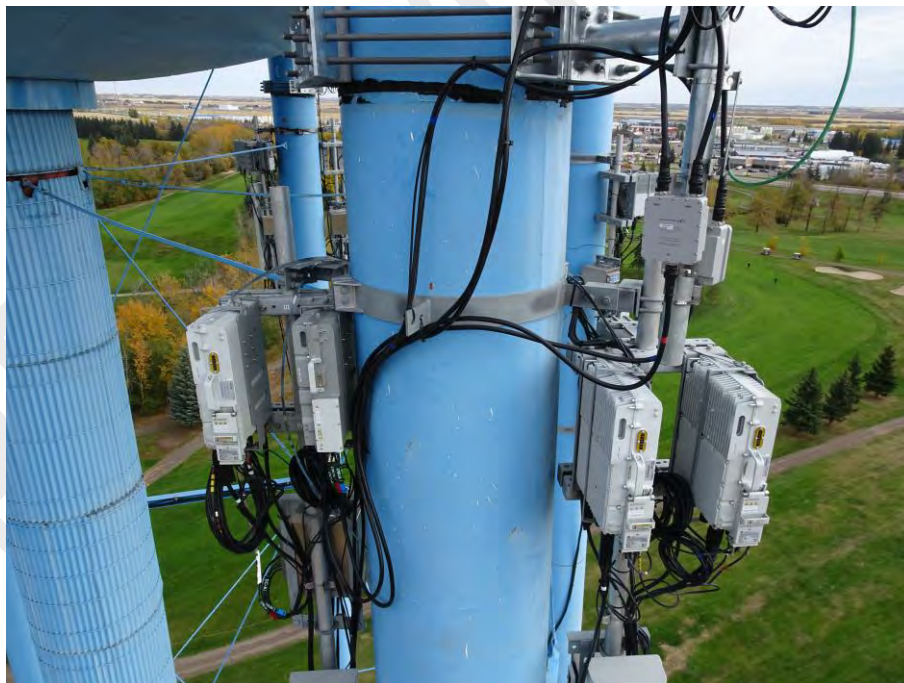
Photo S-12: Antenna hardware connected to column #6
