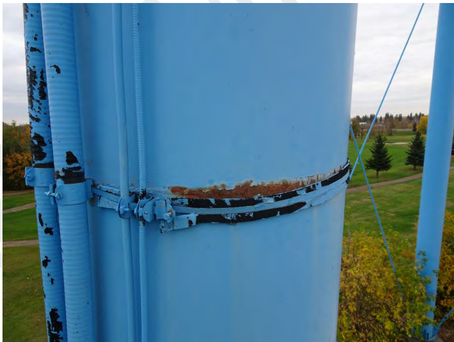
Photo S-6: Rusting and paint wear (Column #2)
