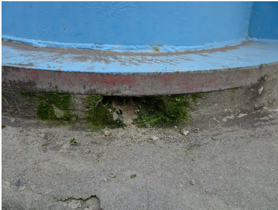
Photo S-3: Deteriorated grout at the underside of the column baseplate (Pier #4)
