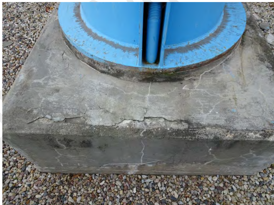
Photo S-2: Plaster has thin cracking throughout and delamination is evident (Pier #3)
