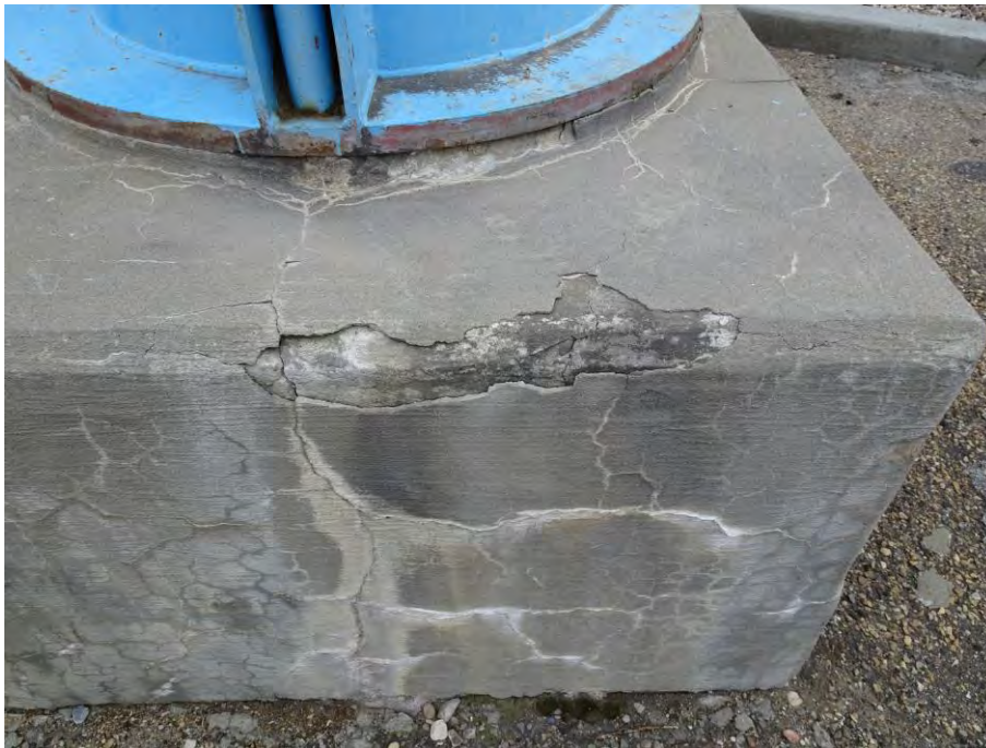
Photo S-1: Cracking evident at column pier #1
