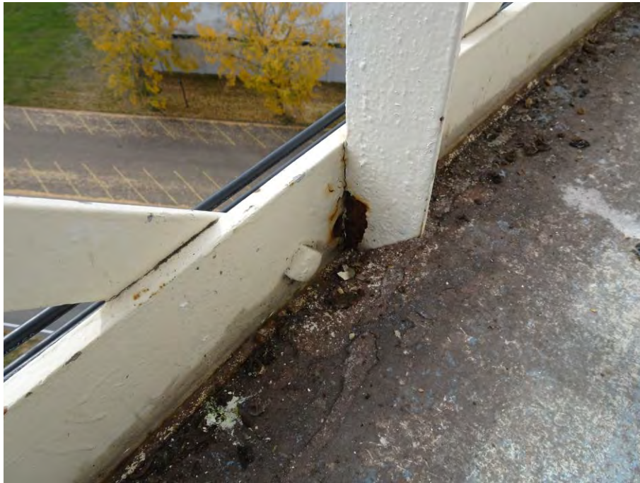
Photo S-9: Spot rusting on handrail and catwalk floor
