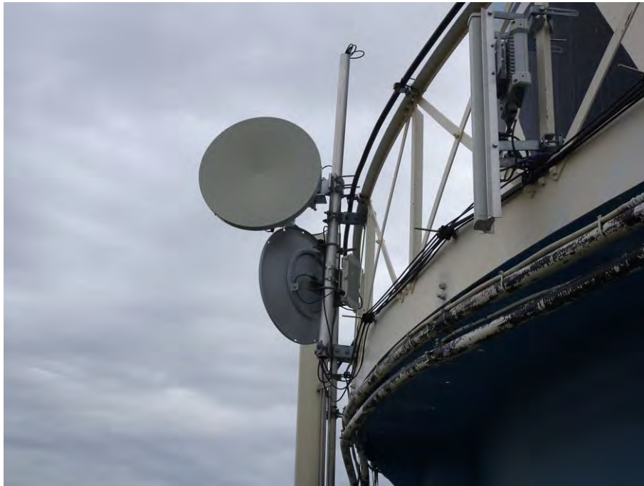
Photo S-13: Antenna hardware connected to catwalk handrail
