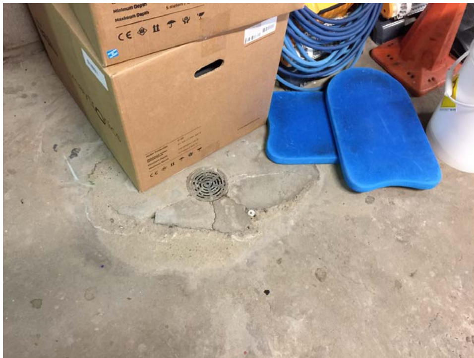
Photo 24: Concrete deterioration around floor drain in mechanical room
