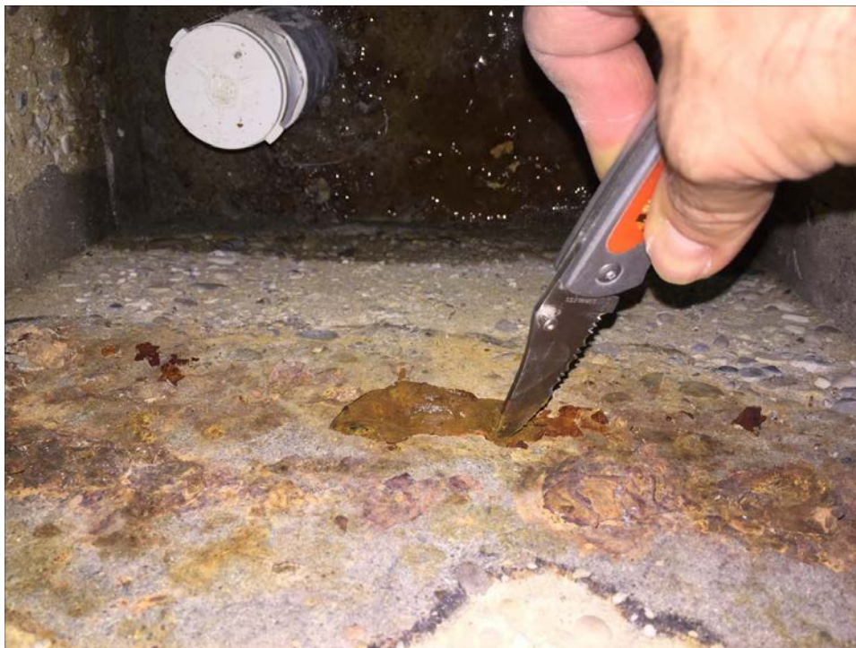
Photo 4: Deteriorated concrete at drain outlet
