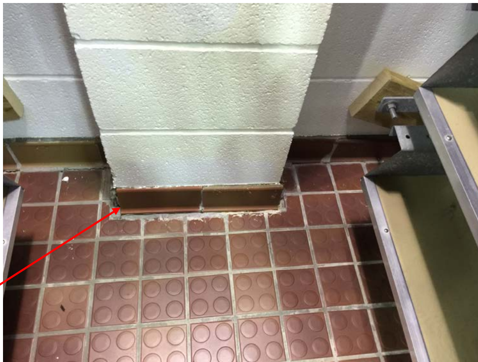
Photo 20: Debonding tiles on vertical upturn along building perimeter
