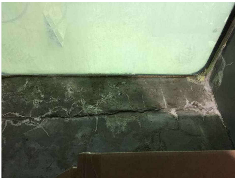
Photo 6: Staining and efflorescence at interior of underwater window – dry side of pool
