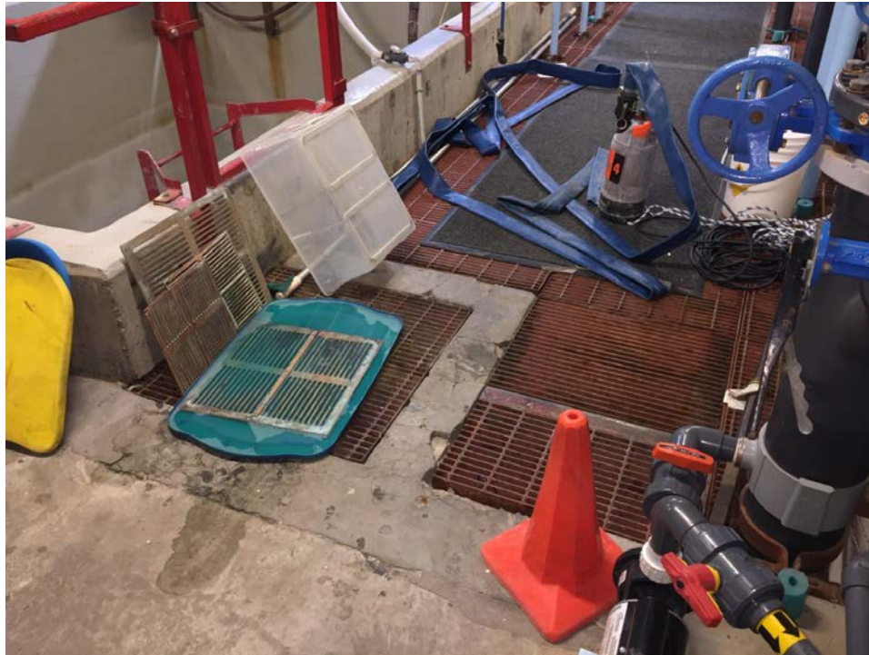
Photo 23: Unprotected concrete slab and metal grating in mechanical room
