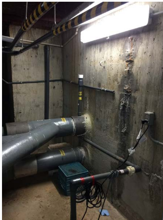
Photo 26: Crack injection work and staining at crack locations opposite mechanical room treatment tanks
