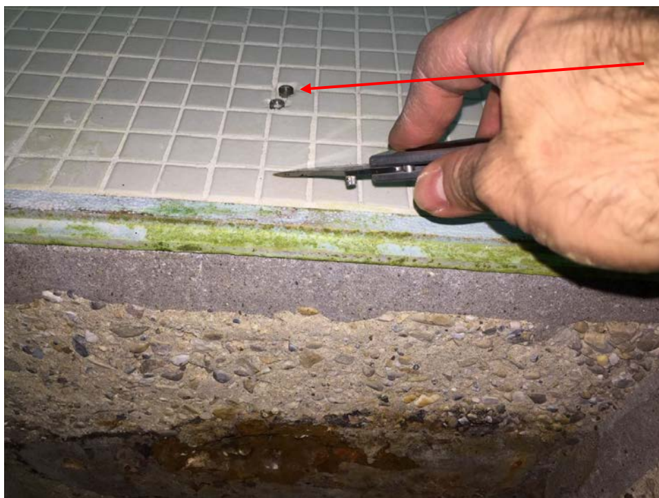
Photo 2: Anchor penetrations through mosaic tiles
