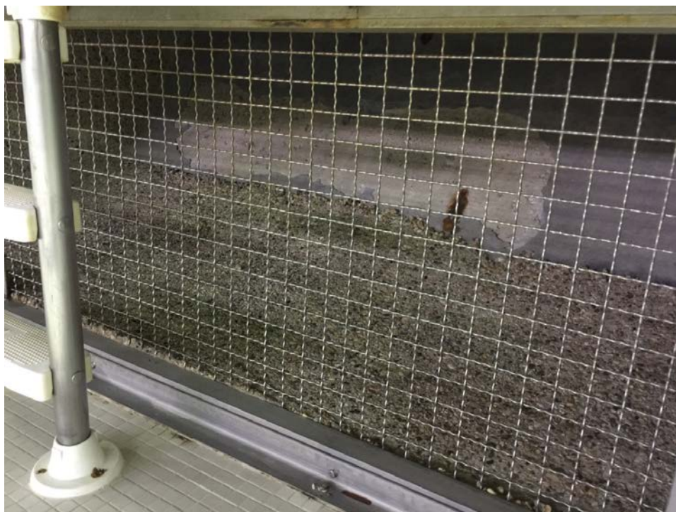
Photo 8: Wave pool chamber – staining and loose concrete
