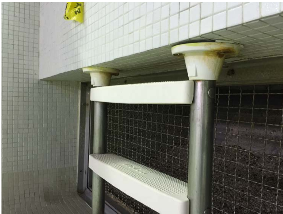
Photo 12: Pool ladder connection – rust staining
