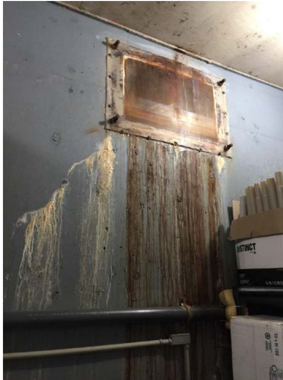
Photo 9: Opposite wall of wave pool chamber – staining and efflorescence at cracks
