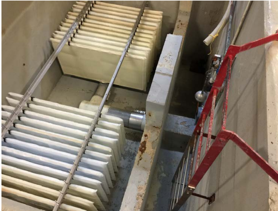
Photo 25: Failed coating and visible concrete deterioration in mechanical room treatment tanks
