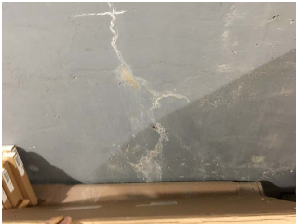
Photo 10: Main pool deep end wall as viewed from below grade corridor – staining and efflorescence at cracks
