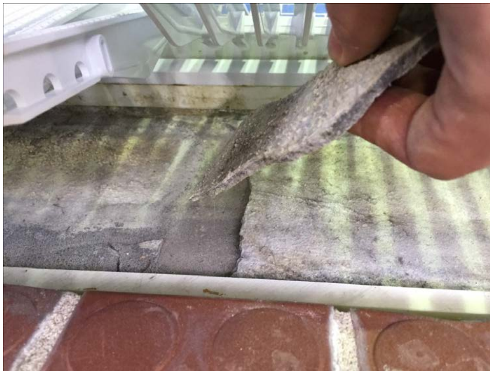
Photo 16: Debonded grout in pool deck trench drain
