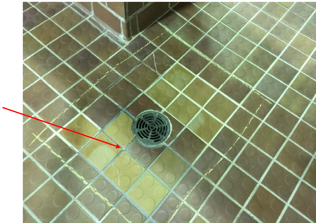
Photo 18: Failing grout at pool deck tiles
