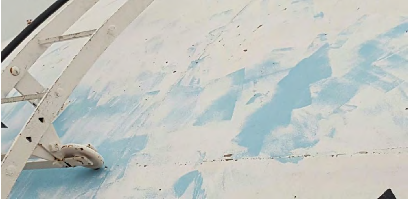
Exposed Mid Coat and small areas of Bare Metal
